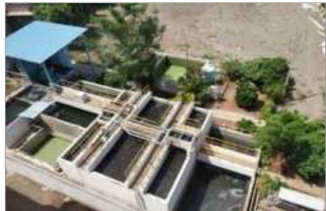
Effluent Water Treatment Plant.
