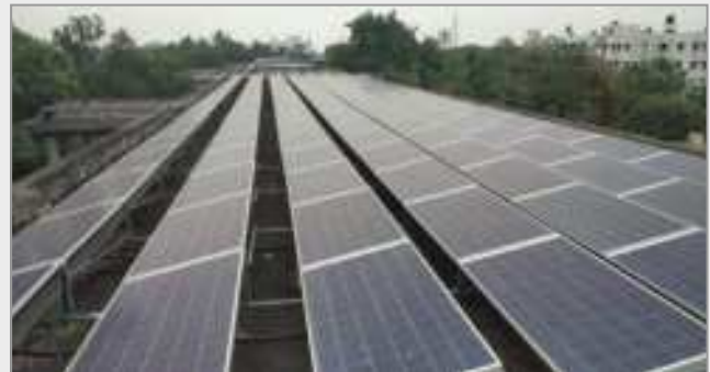
Rooftop Solar Panels
