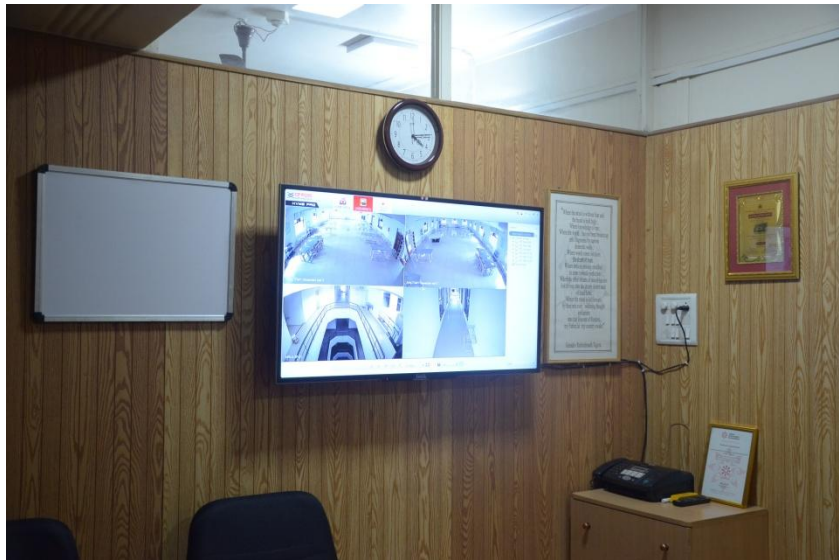
Central Monitor of CCTV feeds at the office of Principal
